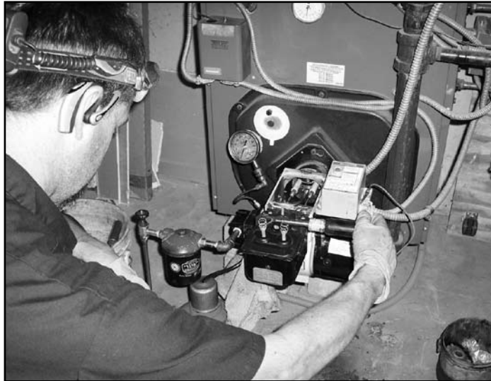
Our technicians are working hard on annual tune-ups to improve your heating efficiency.
